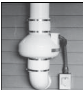
The exhaust fan creates vacuum to draw radon and other toxic gases from the water storage chamber.
