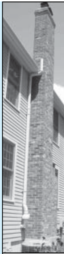
Example of vent pipe installation.
