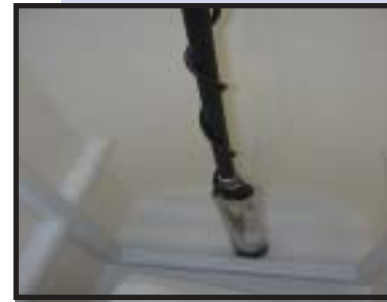
Submersible pump to re-pressurize product water to 64 psi up to 20 GPM.
