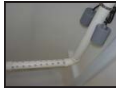
Bubble up blower pipe moves 64 to 80 cubic feet of air per minute only on fill cycle.
